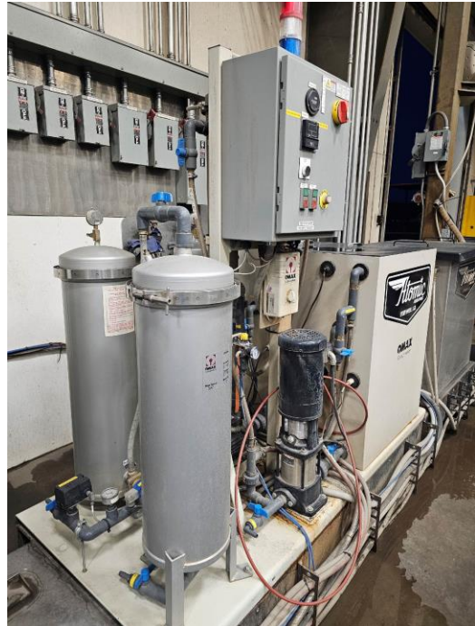
Water filtration system
